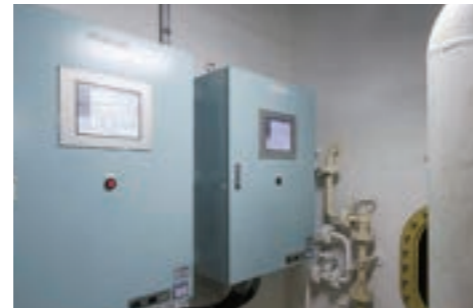
Control panels in engine room
